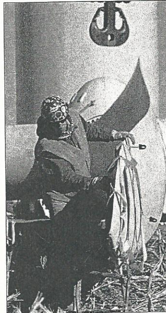
Rodney Borkenhagen, a union iron worker, secures protective webbing over the tip of a 122-foot wind turbine blade before it is lifted into place on the Forward Wind Energy Project near Lomira on Nov. 1, 2007. (AP File photo/The Reporter, Justin Connaher)
