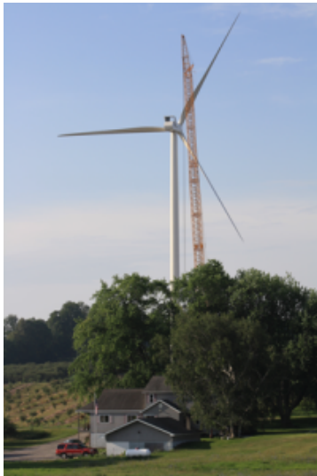
An industrial-scale wind turbine during installation near the Shineldecker home in Mason County, Michigan.
